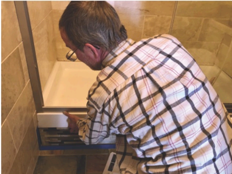
Cunningham installs glass and ceramic subway tiles in a tight bathroom space. Photo by Susan Schaefer
